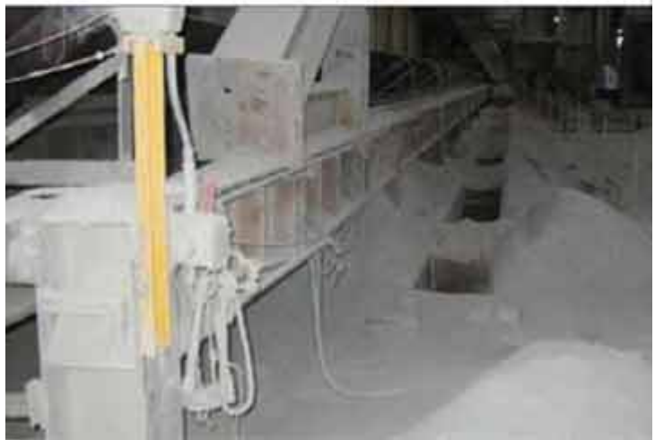
Report by international commission organized by Maquiladora Health & Safety Support Network documented how dust collectors have been disconnected by the company (top), leading to huge accumulations of deadly silica dust as well as dangerous holes in the floor. (Photo: MHSS)
