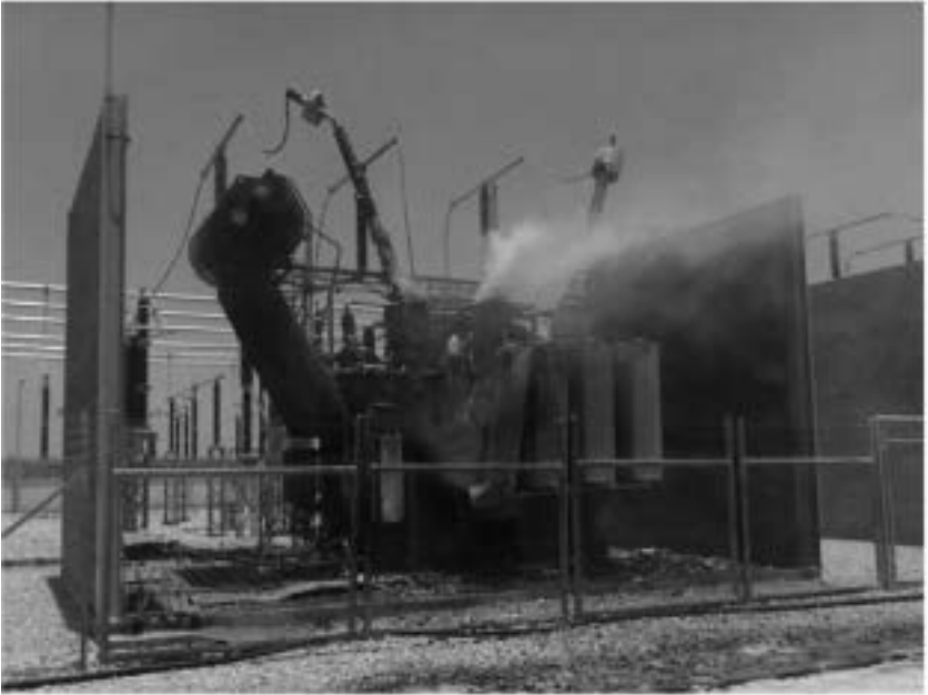
8.5 The Gaza electricity generation facility destroyed by an Israeli air strike on 26 June 2006.
